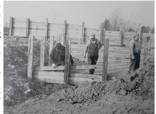
Bob Pickworth, Jim Sheffield & an unidentified man constructing an animal waste holding structure in 1972.
