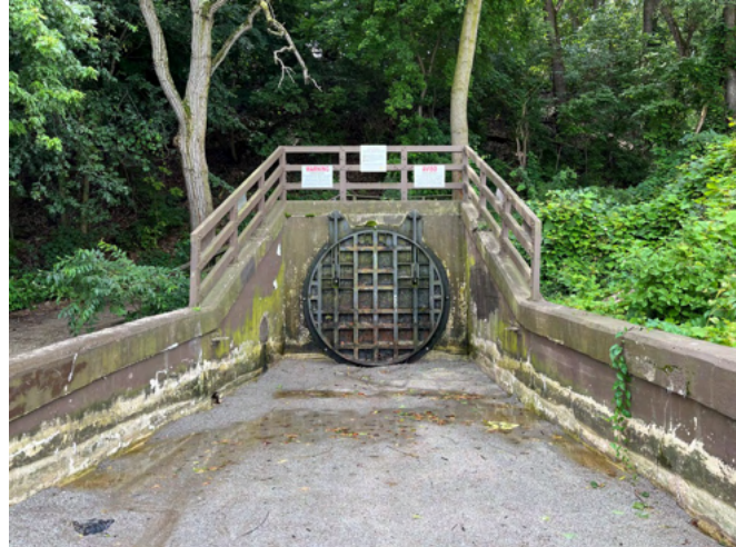
Combined sewer overflow outlet.
