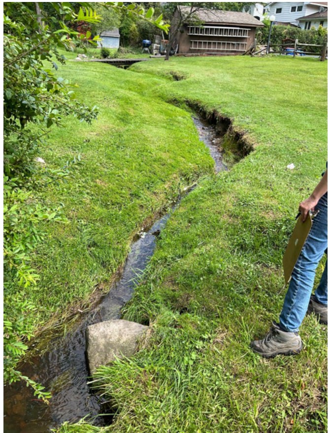
Example of stream cutting and erosion.
